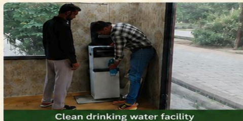
Clean drinking water facility
